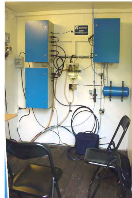
From an integrated measuring station in Poland
